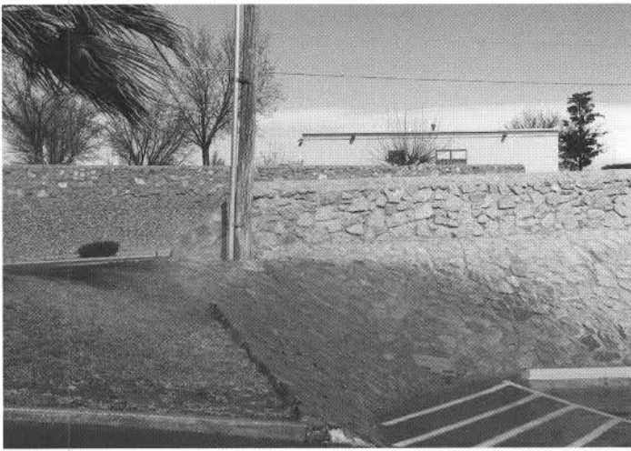
FIGURE 7. Two types of stone are commonly used in walls and hardened slopes in southern New Mexico and west Texas. In the background rock in the sloping surface is gray Vado Andesite. In the foreground and to the right are gray-to-yellow Hueco Limestone blocks. A yellow color (here as light gray) is developed on weathered joint surfaces.
