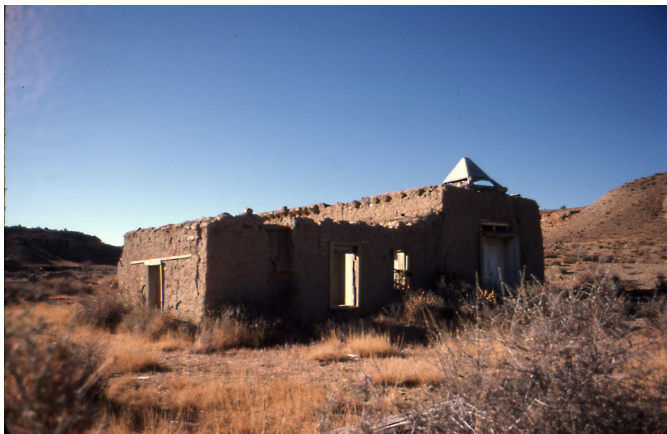
FIGURE 2.67. Catholic church at Guadalupe (photo taken in 1978). Since then, the steeple has fallen (or was placed) on the ground.
