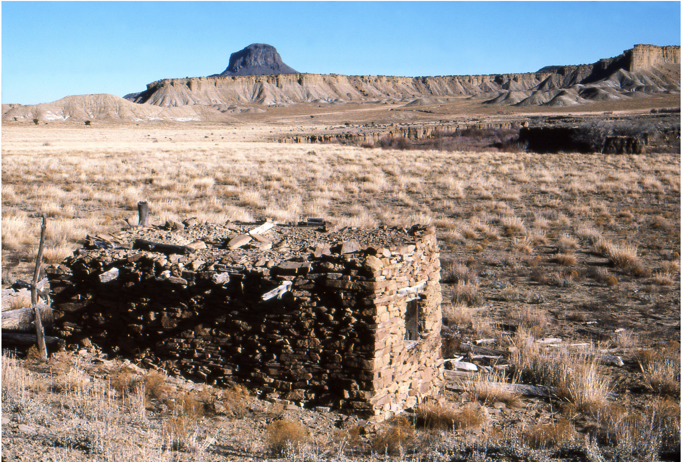
Stone-masonry cabin likely built by Hispanic farmers during 1880–1950. The cliffs across the Rio Puerco are capped by the Dalton-Hosta sandstone tongue. The impressive Cabezon neck stands on the left. View is to the east.
